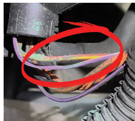
The badly damaged wire (circled) was very obvious, and was easily repaired
