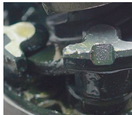
Crystallized stop-leak agent thickened this oil, creating visible grit in the compressor
