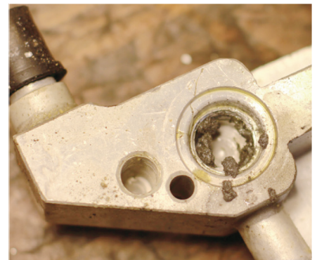
Visible soiling at the condenser inlet
