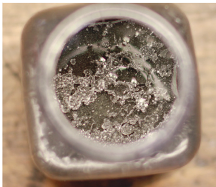
Oil drained from a seized compressor. The visible contaminations are spread in the entire system, including the condenser
