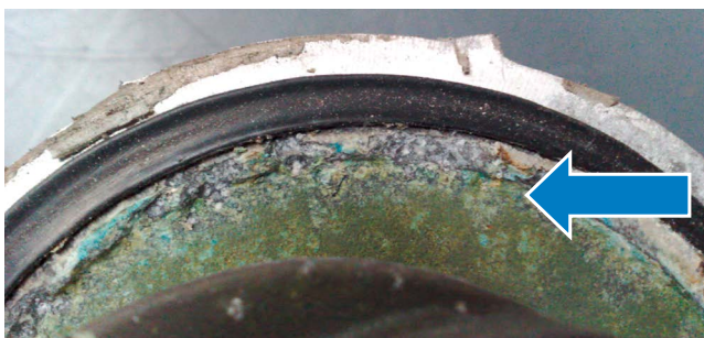
Unsuitable cooling liquid has led to corrosion and leakage
